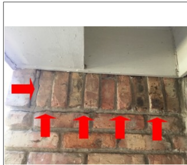
Left side front entrance separation
