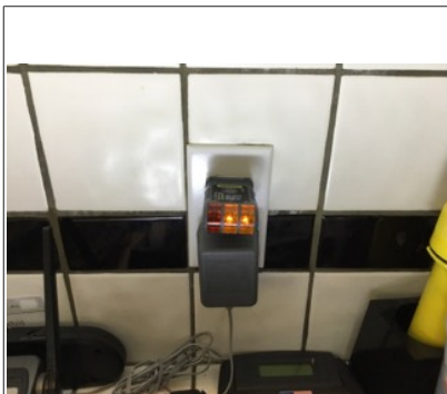
Kitchen receptacles not gfc protected
