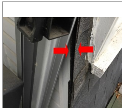
2 layers of roof covering
