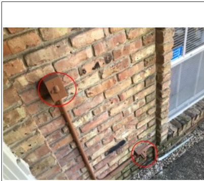
Front entrance exterior outlet non GFCI protected and switch not functional
